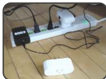
INSTALLED ADVANCED POWER STRIP & SMART PLUG TO REDUCE PHANTOM ENERGY DRAIN
